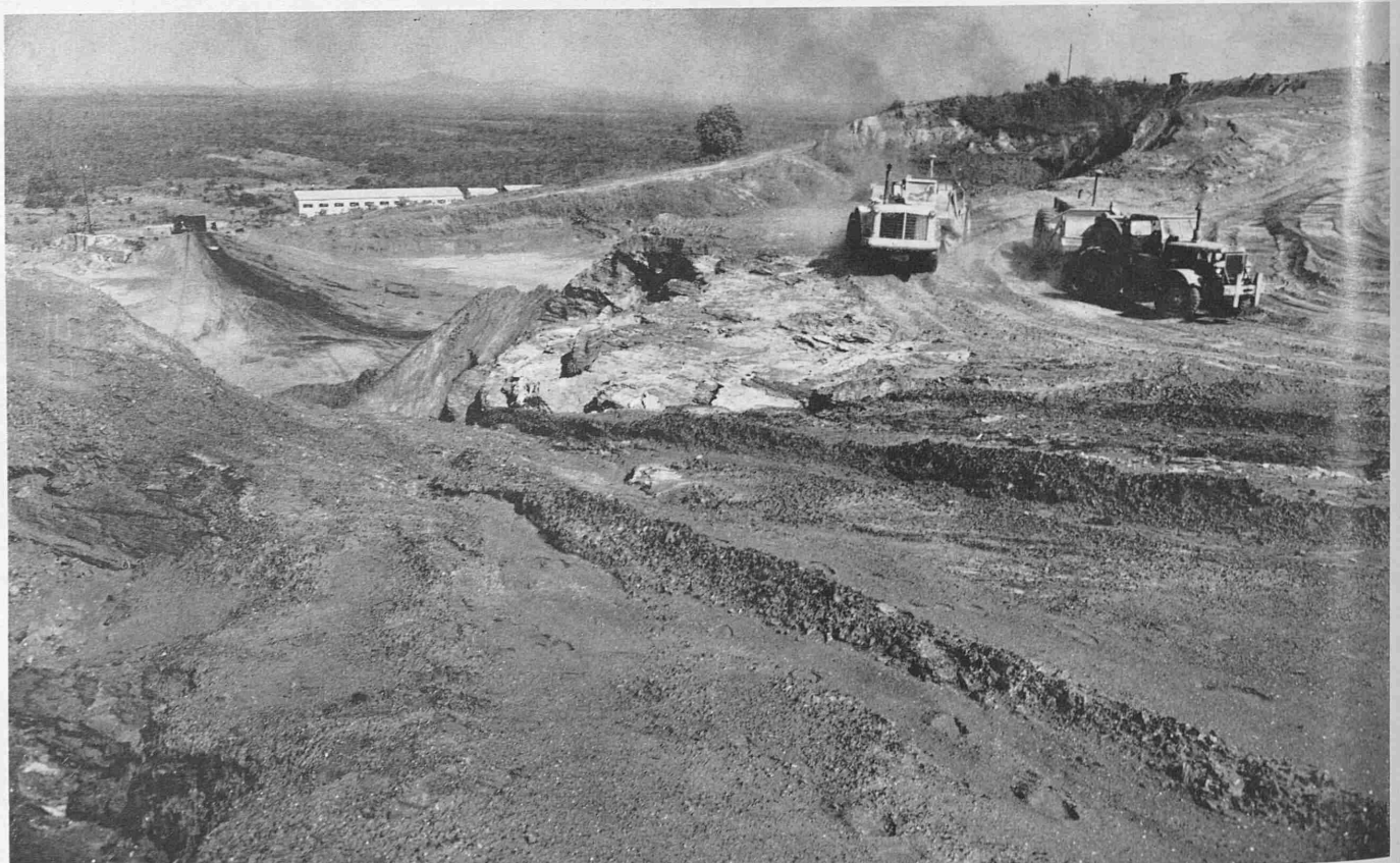
A general view of the workings at the iron ore mine at Marampa. Euclid twin-power scrapers are removing the ore. Over the ridge in background is the roof of the concentrating mills of the Sierra Leone Development Company. The ore deposits were discovered in 1927 and first shipments made in 1933
