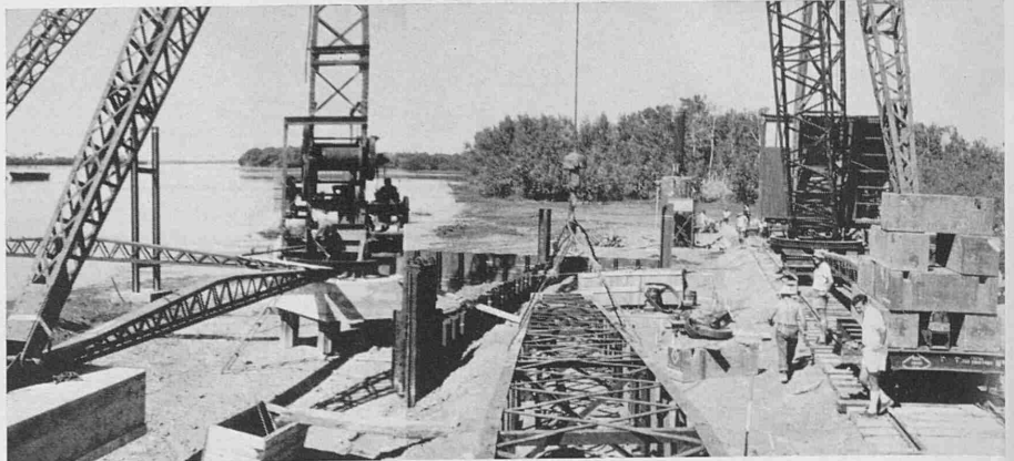
The construction of the first stages of the extensions at Pepel, from which the iron ore is shipped. All the modernisation work, being undertaken by Taylor Woodrow, should be completed by 1964
